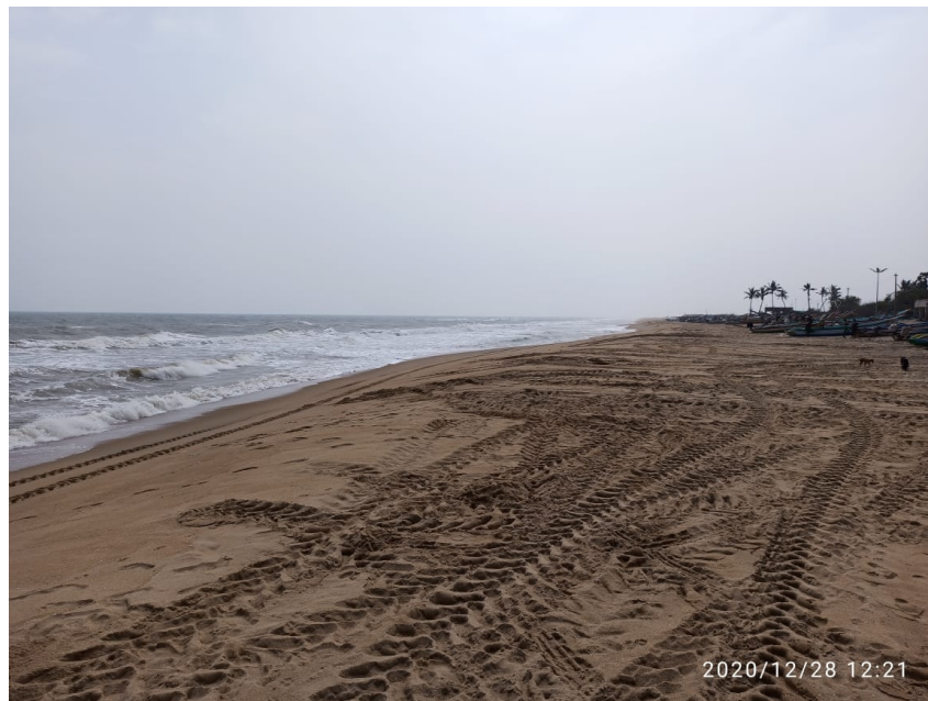
Fig. 2 Site Condition and Erosion at Uyyalikuppam village
